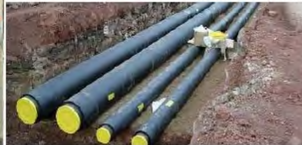
NEW HEATING AND COOLING SYSTEM
